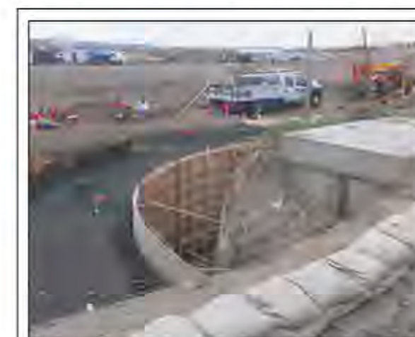
Toxic contamination was discovered while constructing this storm drain at the Portola High School site in November of 2014.
