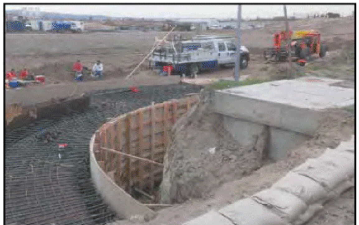
Toxic contamination was discovered while constructing this storm drain at the site of the new High School. The discovery and subsequent findings were not disclosed to the public.
