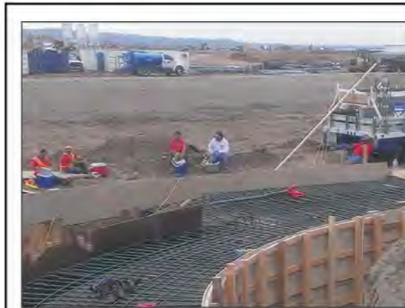
After discovery of toxic contamination while constructing this storm drain at the Portola High School site in November of 2014, the City’s environmental consultant reported that he expected DTSC to immediately order new testing for toxic petrochemicals. The expected testing never happened.
